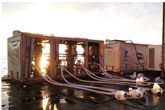
Figure 4. LNG transfer system trucks/Iso-container.
